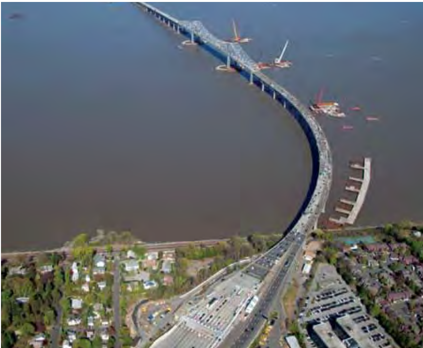
Tappan Zee Constructors installs the main span piles for the New NY Bridge.
