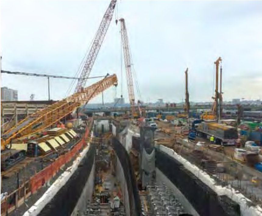
Construction of the tunnel box under Hudson Yards for Amtrak's Gateway passenger rail tunnels
