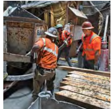
Second Avenue Subway, 86th Street Station: street-level crane lowering concrete bucket for concrete pour
